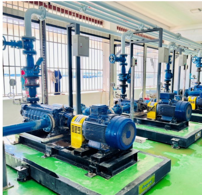
Figure 3. Sitagu Water Pumping Station, Sagaing, Myanmar.
